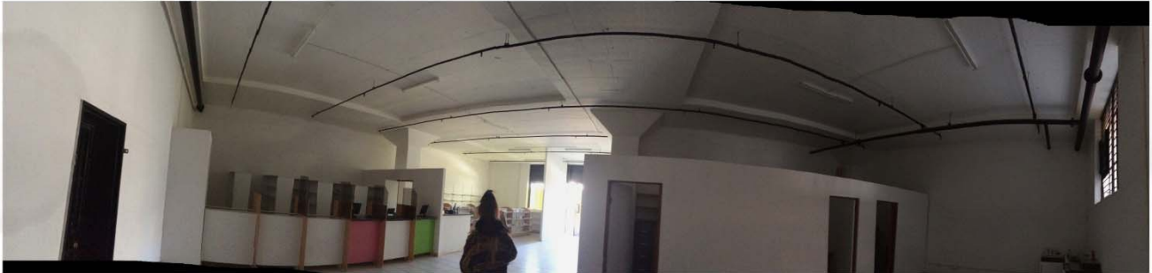
Industrial structure. Roof articulations in the concrete slab. Neutral finishes. Existing systems: interior drywalls, chipboard shopfitting, duct, fire sprinklers and tube lighting.
