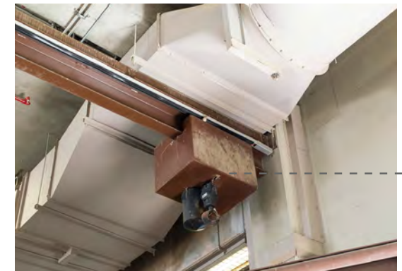
Figure 8. 7 Block and tackle running along steel beam used to raise elephants in emergencies, at the Smithsonian Zoo (Author, 2016).
