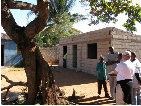
FIGURE 9: A typical new house construction with two rooms, built from concrete blocks with a reinforced concrete ring beam cast in situ, and with roof covered with corrugated iron sheets.
