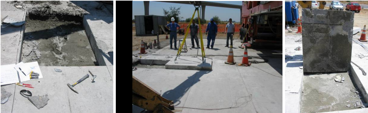
Figure 11. Investigation of void under the slab in Section 2
