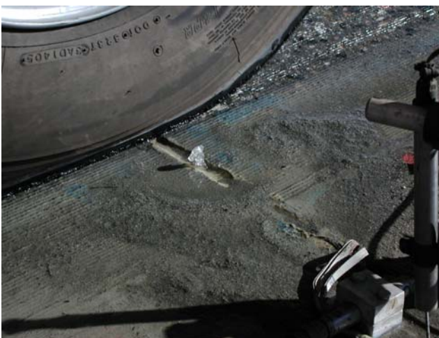
Figure 10: Water pumping from a joint during the wet cycle
