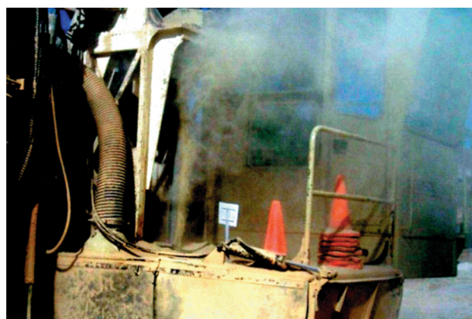
Figure 5. Dust escaping the sealing ring where the drill stem enters the drill deck
