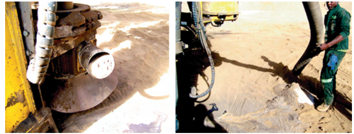
Figure 7. Blocked dust collector pipe between shroud and cyclone
