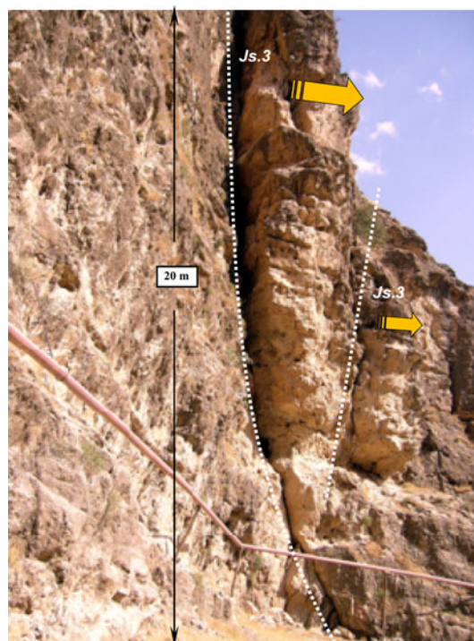
Fig. 19 Toppling failure along joint set.3 on the left bank of the Seymareh River valley
