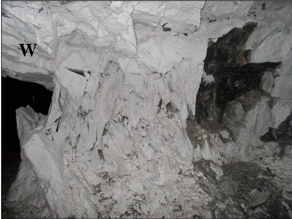
Figure 8.33: Continued scaling and dilation of the western side of pillar P2 (down-dip view from the holing above the pillar). The photograph was taken on 6 May.
