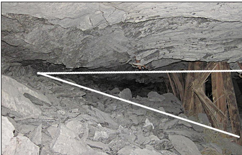
Figure 1.7: Example of pillar bursting. The scattered pillar material was ejected into the siding. The white lines indicate the scatter relative to the stopping width. Timber elongates indicate dynamic loading as a result of the event.
