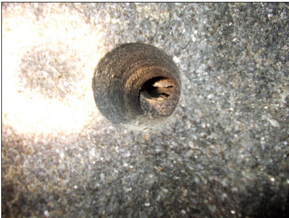
Figure 8.36: Movement along the borehole drilled through the pillar from the western side. The photograph was taken on 6 May.
