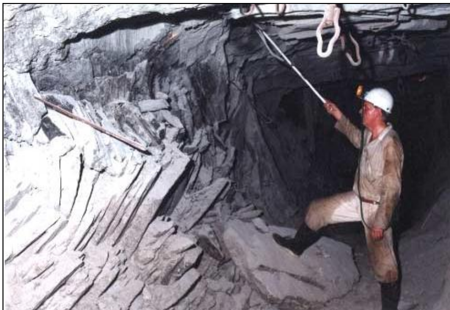
Figure 5.17: Crush pillar directly adjacent to a gully (with no siding) in a Merensky stope at 700 mbs (after Naidoo et al, 2002).
