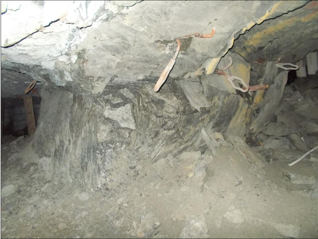
Figure 8.38: Fracturing along the bottom west and western surface of pillar P4. The photograph was taken from the holing below the pillar on 6 May. The pillar extensometer is also visible in the photograph (steel pipe casing protruding from pillar).
