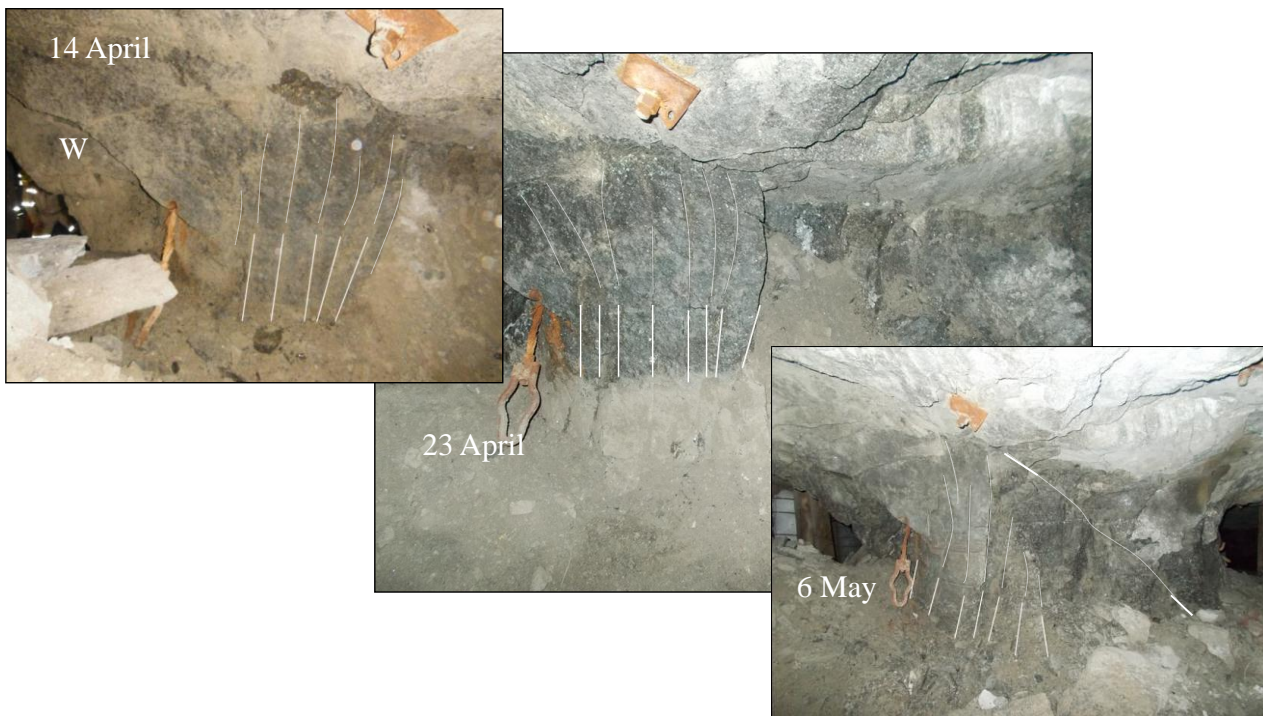
Figure 8.37: Fracturing along the top western side of pillar P4. The photographs were taken from the up-dip holing. Also note the diagonal fracture in the photograph labeled 6 May.
