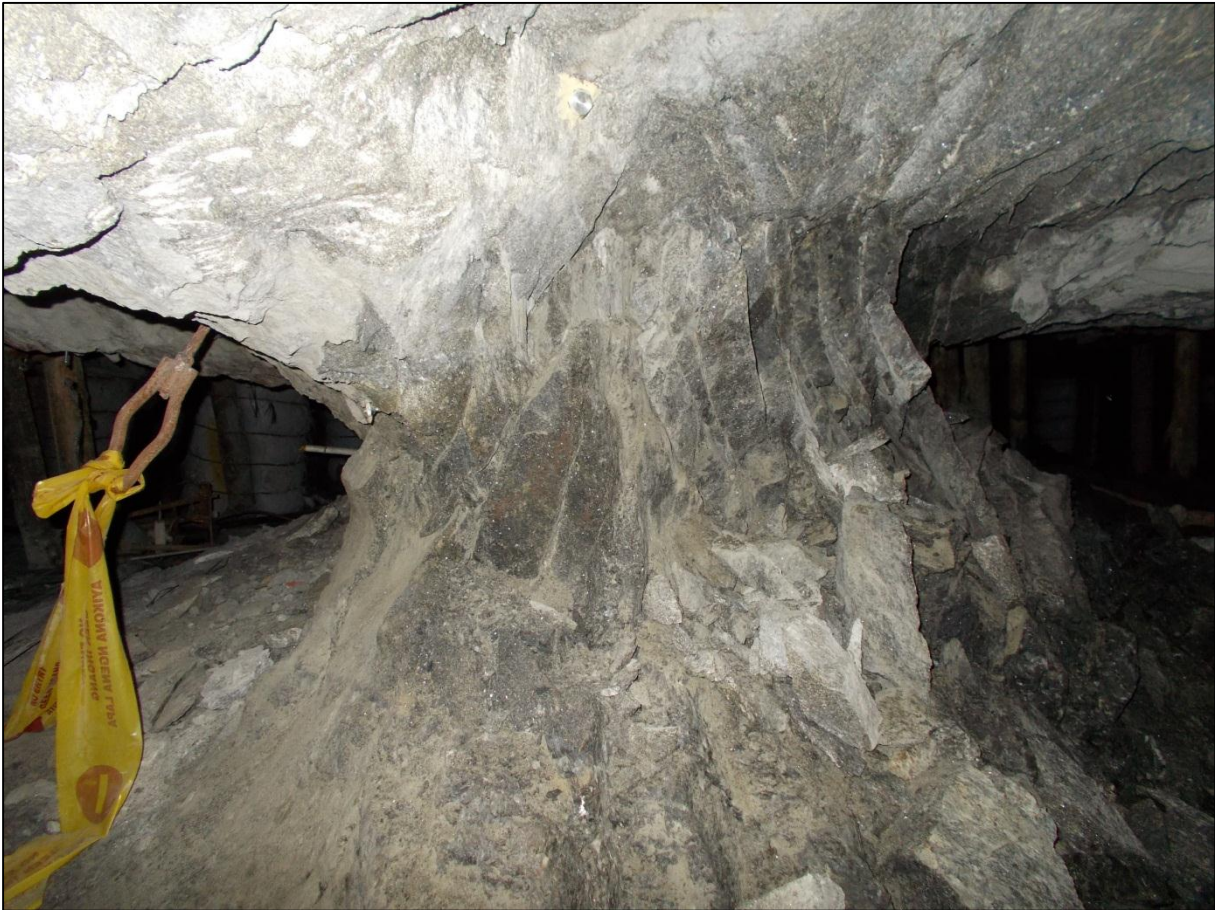
Figure 1.4: Photograph of a crush pillar from a trial site on Lonmin Platinum.
