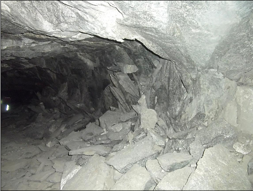
Figure 8.17a: Anorthositic pillar sidewall scaling.
