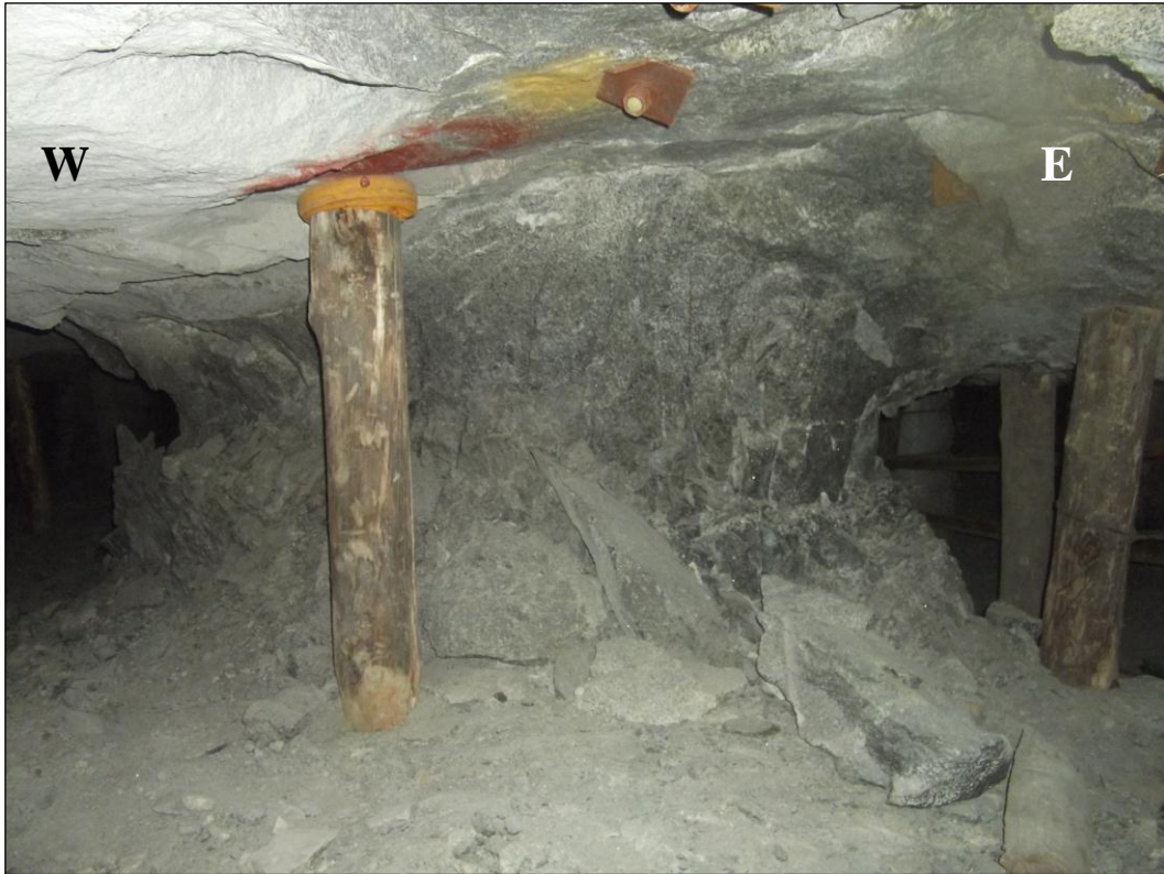
Figure 8.12a: Pillar scaling towards the west. Photograph of the up-dip side of pillar 18.
