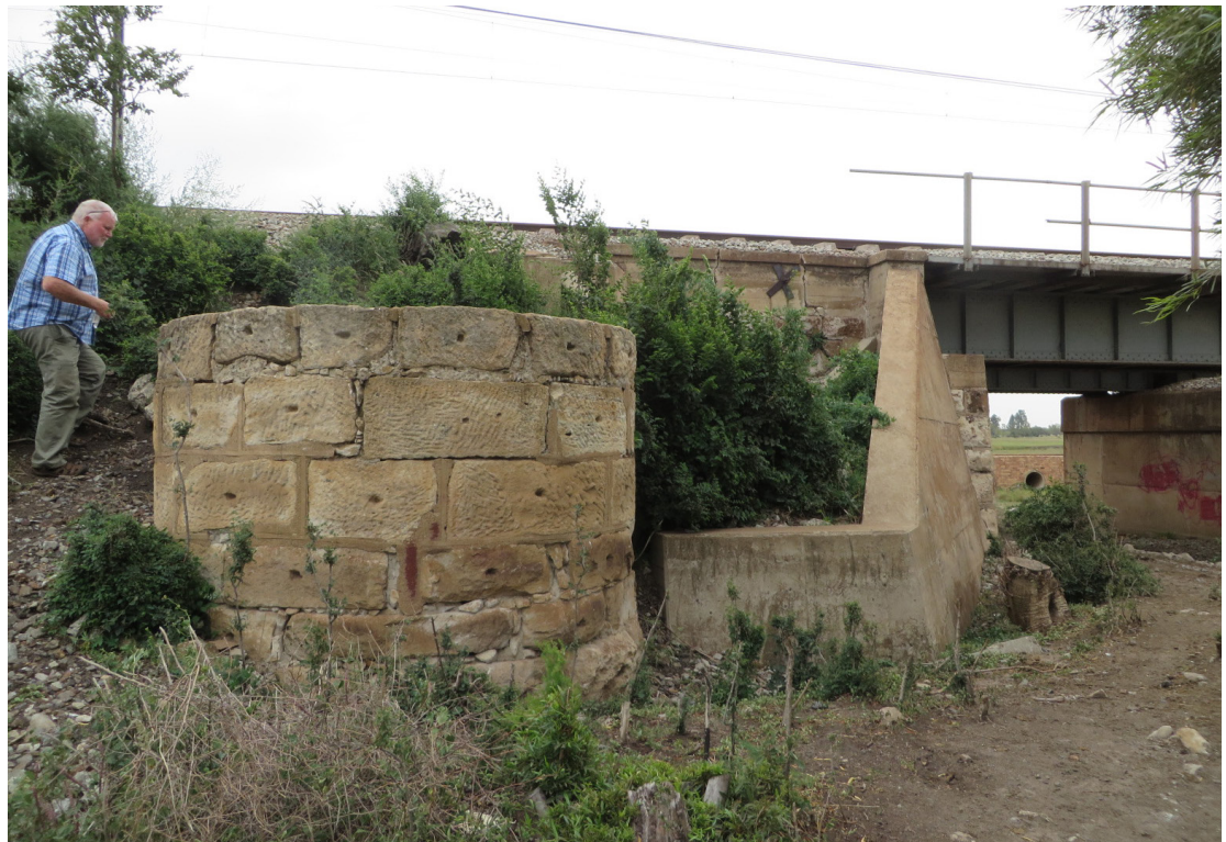
05.4: The well at Koekemoerspruit Bridge (NZASM_SWL_022) being inspected by Fisher on 2016 04 06. This unique structure deserves designation as a listed heritage resource.
