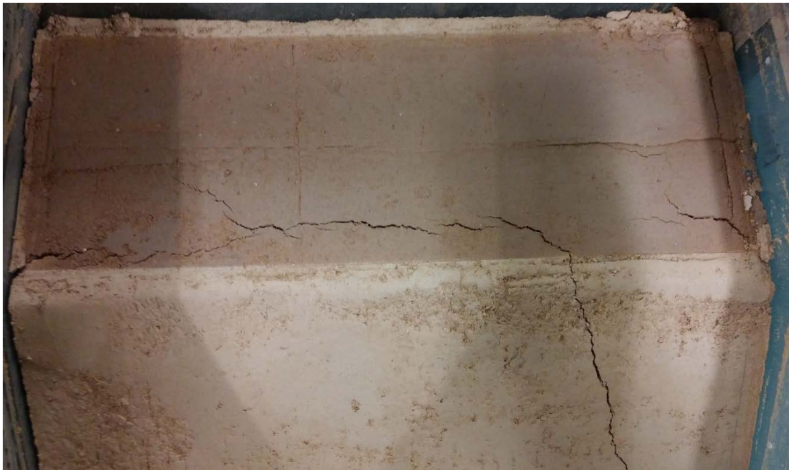
Figure 4.29: Cracks across the top length of the embankment formed during Test B6 (23.0 % MC)
