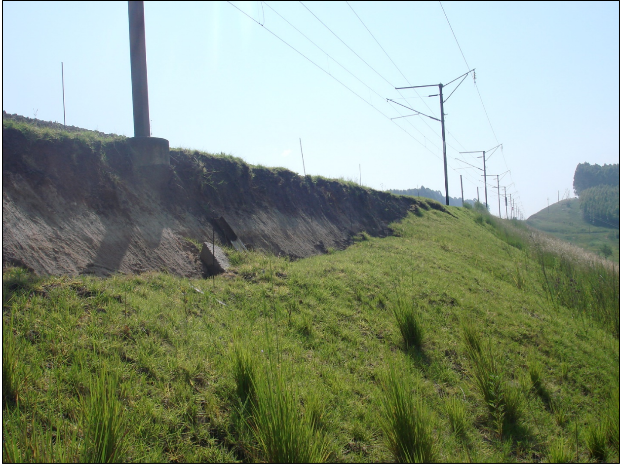
Figure 2.5: Embankment slope failure on the Ermelo-Richards bay line (Transnet Report, 2007)
