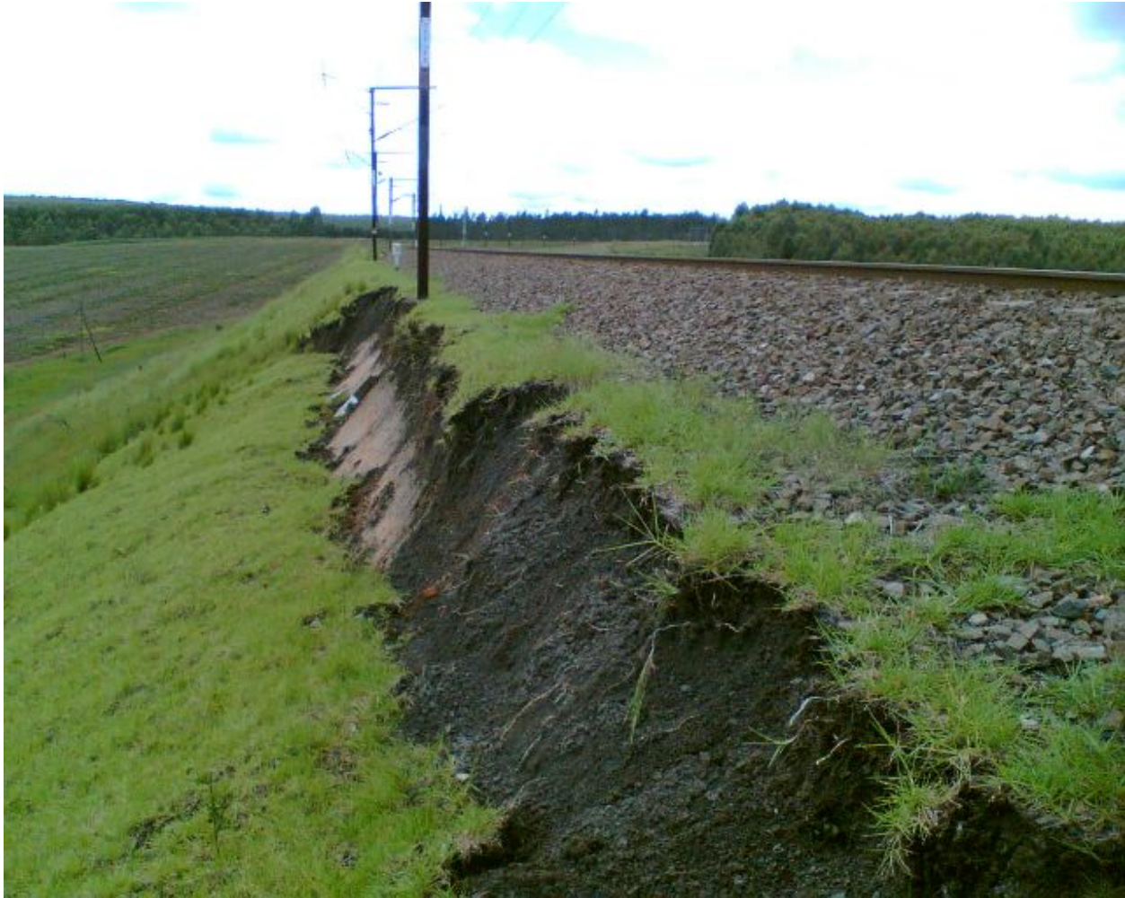
Figure 2.6: Embankment slope failure on the Ermelo-Richards bay line (Transnet Report, 2007)
