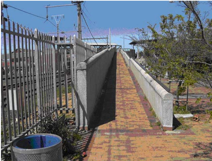
Figure 3. This photograph taken at Mowbray Transport Interchange in Cape Town shows the ramp available to SNP's. The problem with this ramp is that there is no landing and with the gradient used, a landing is needed.
