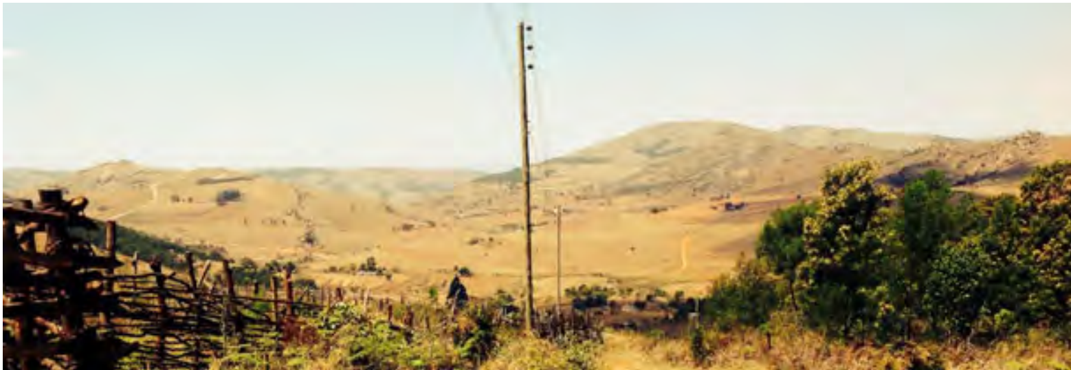
1.028 Electric power lines funded by the Chinese government span the landscape of Mabeleni. This sparsely populated rural informal settlement is developing into an urban area – 2014.
