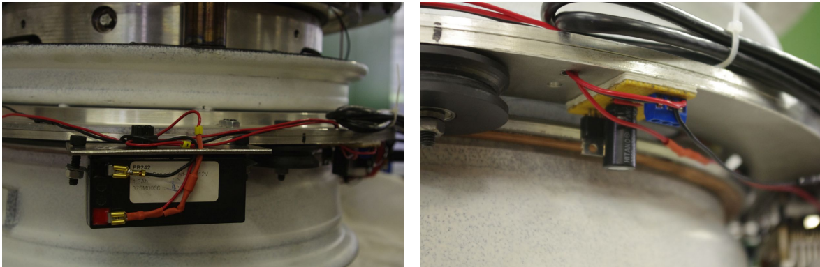
(a) The battery used to prevent power interruptions.
