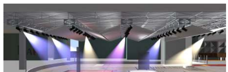
Figure 4.6.14. View of suspended lighting system
