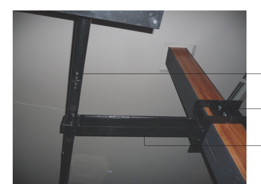
Secondary support - supports projector System fixed to column with expansion bolts Main horizontal brace
