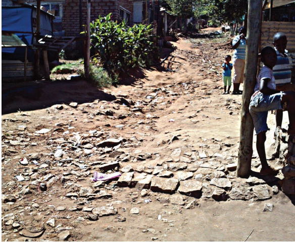
Figure 24 Erosion along a path running down the mountain side (Author 2015)
