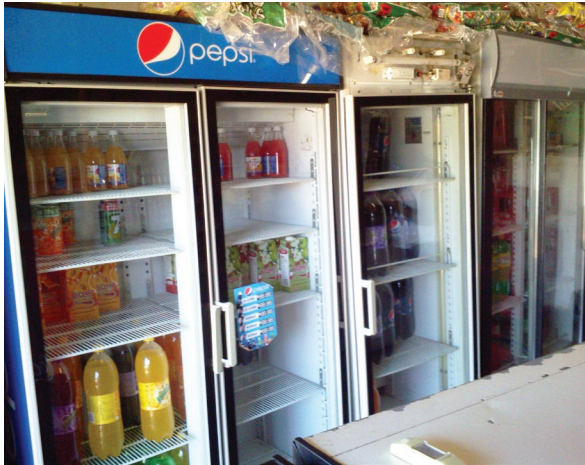
Figure 6 Supermarket fridges used to cool non-perishables instead of fresh produce (Author 2015)
