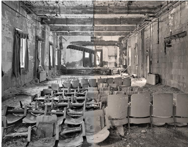
Figure 3.2 : Photographic illustrations of decay in architecture (Author, 2015).
