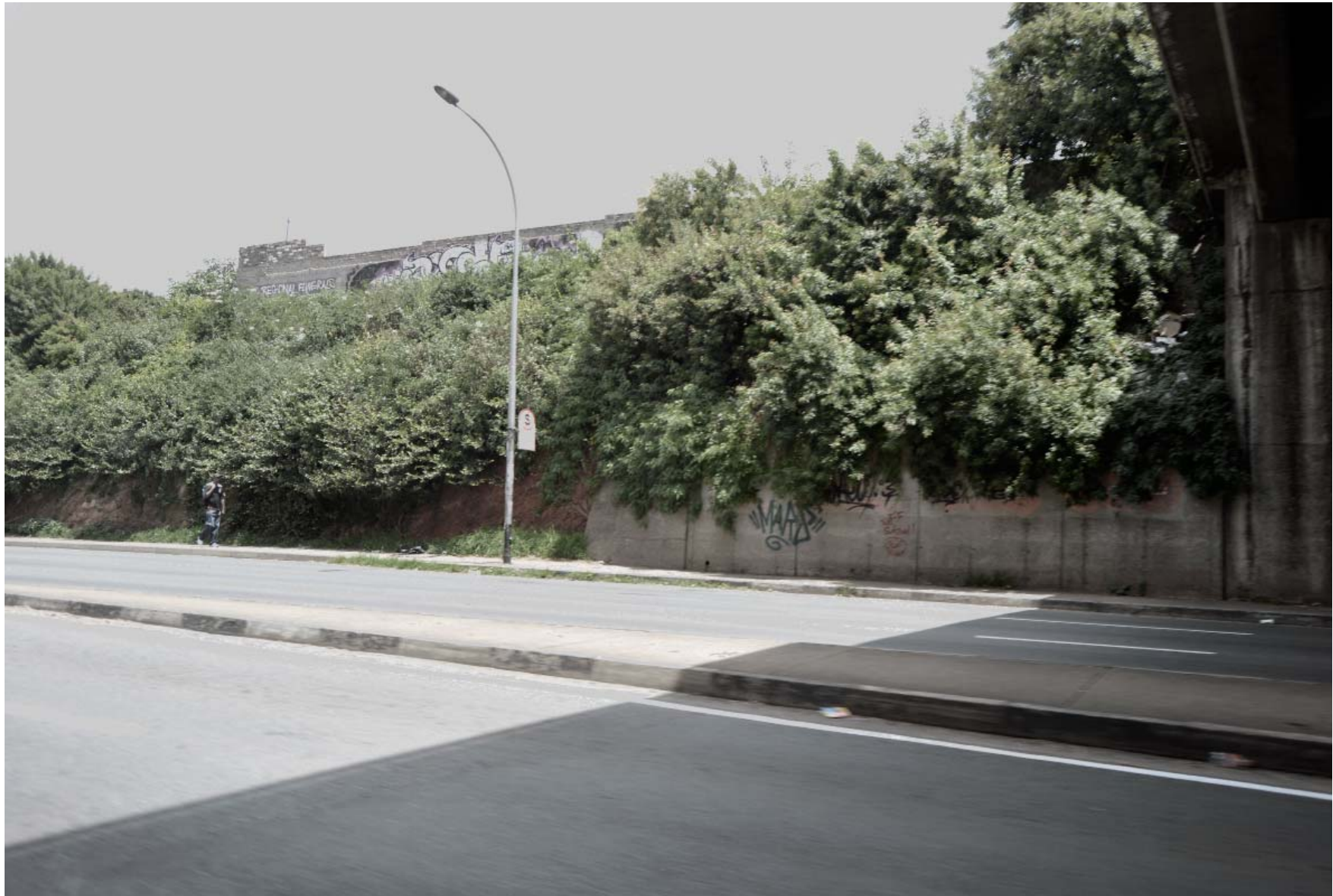
fig 4.12. Ridge, Concrete Bridge and Nature come into conflict on Joe Slovo drive. (by Author, 2015)
