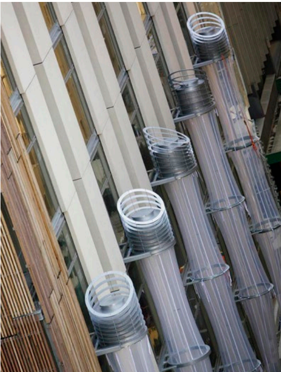
Figure 8.28: Photograph of the air inlets at the top of the cooling towers, Photo by Melbourne Council House, Australia (Ecofriendly architecture 2014)
