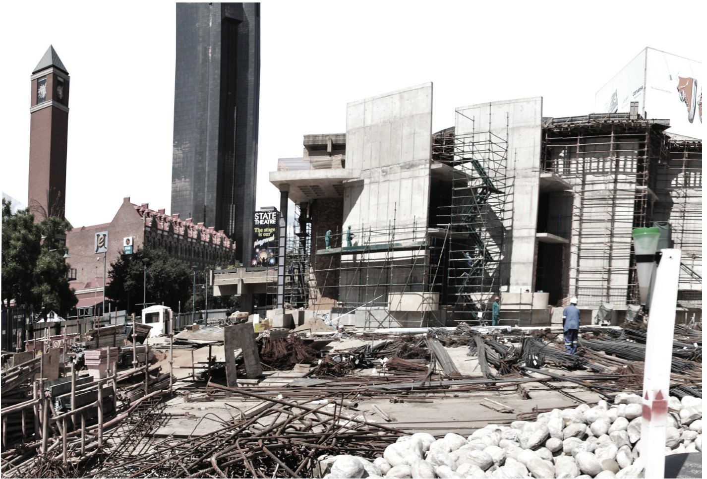
Figure 3.7 Construction of the Women's Living Memorial on Lillian Ngoyi Square, March 2015. (Source: Author, 2015)
