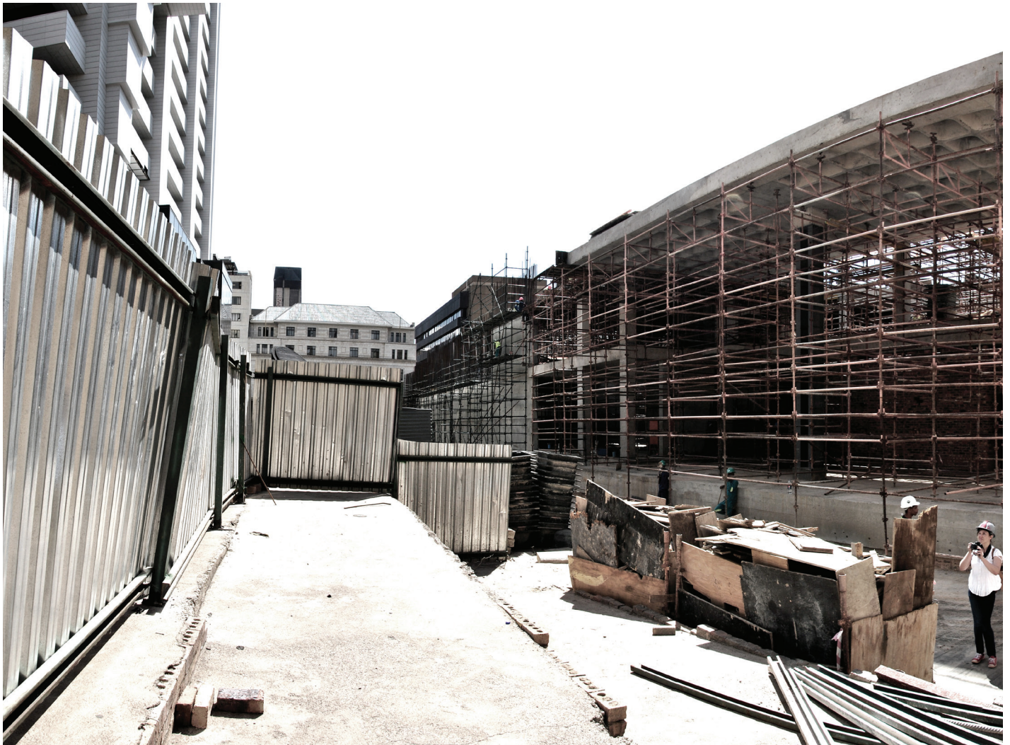
Figure 3.8 Uncomfortable alleyways are created between the new memorial and the State Theatre and ABSA Tower. (Source: De Verediciis, 2015)
