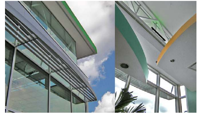
Figure Appendix B5: Exterior & interior views of roof overhang, sunshades and energy efficient insulated glazing (WBDG 2014)
