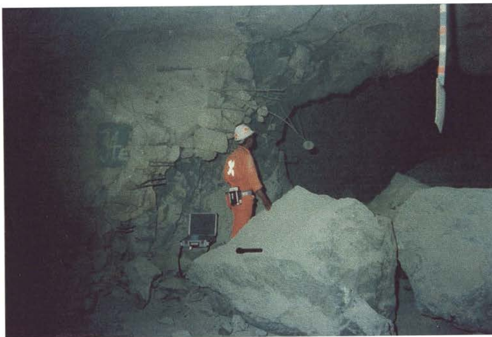
P.A.5. DS3 on Damage Scale. Damage to steelwork and underlying rock in bullnose on 630 metre level (RMR 52).
