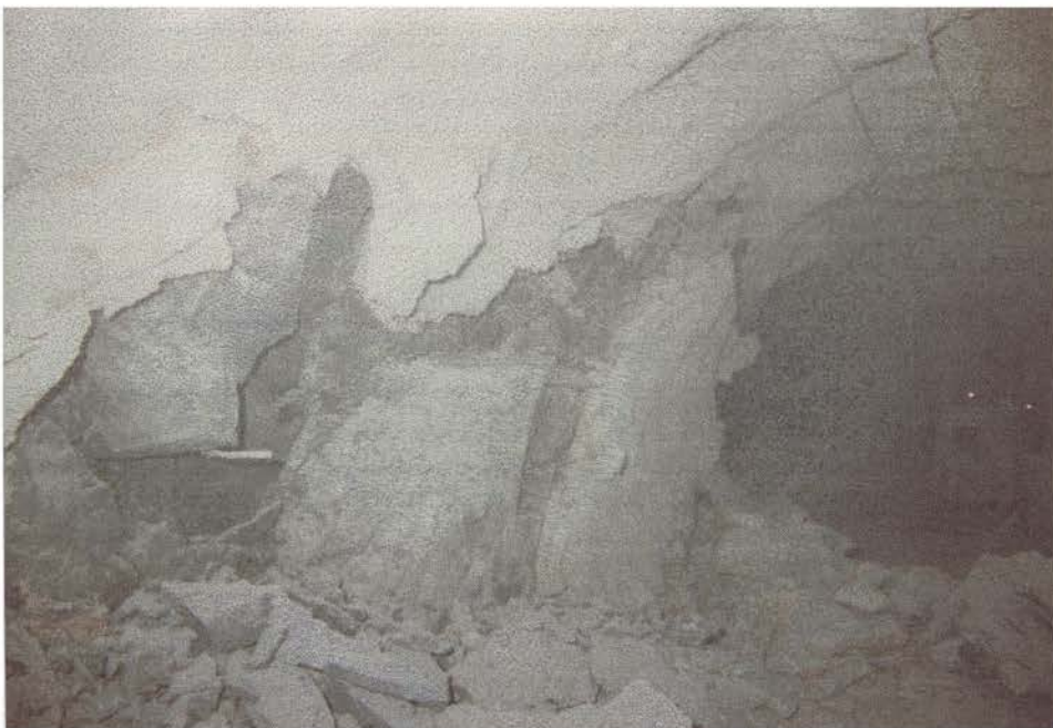
P.A.7. DS4 on Damage Scale. Extensive damage to support and rock on 630 metre level in Tuffisitic Kimberlite Breccia (RMR 50).
