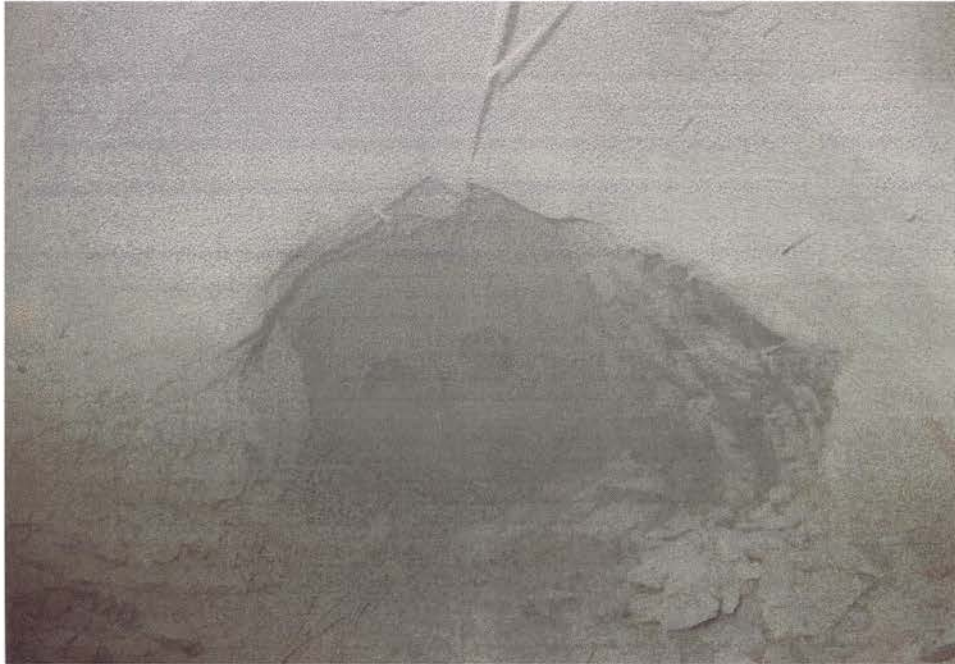
P.A.8. DS4 on Damage Scale. Extensive damage to support in Tuffisitic Kimberlite Breccia on 630 metre level as a result of induced fracturing after undercut has passed overhead.
