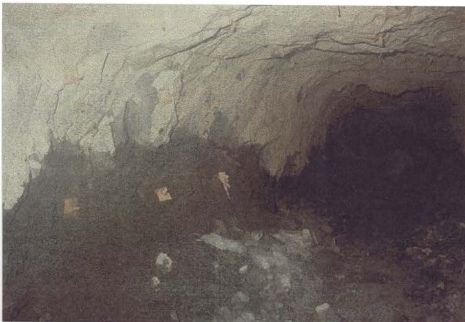
P.A.11. DS5 on Damage Scale. Water damage results in decomposition and complete loss of rock mass strength (RMR 52) Location: 30 Main on 630 metre level.
