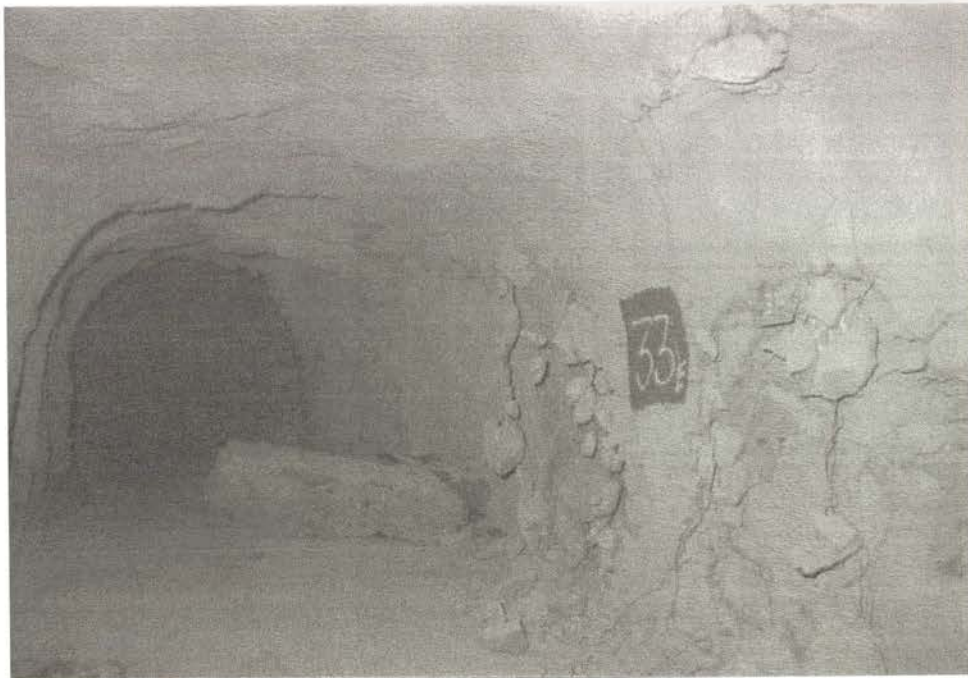
P.A.4. DS2 on Damage Scale. Extensive cracking of rigid shotcrete lining on 630 level after undercut has passed overhead (RMR 50).
