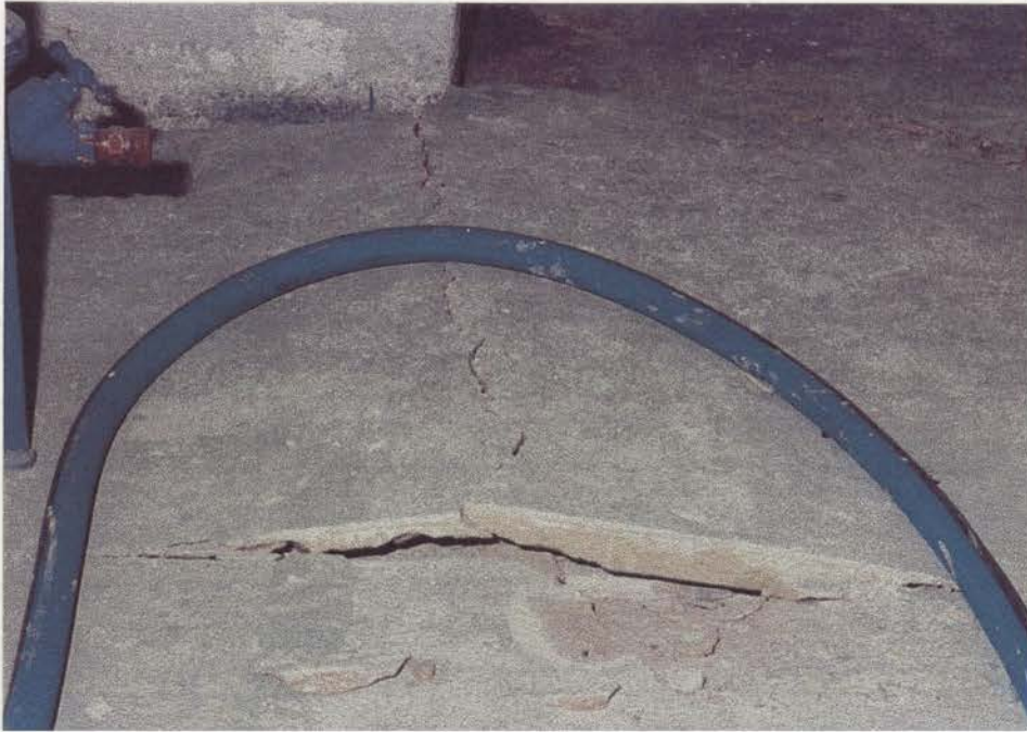
P.A.2. DS1 on Damage Scale. Concrete damage in refuge bay 60 metres from abutment on 630 level as a result of movement on joints in norite (RMR 45).
