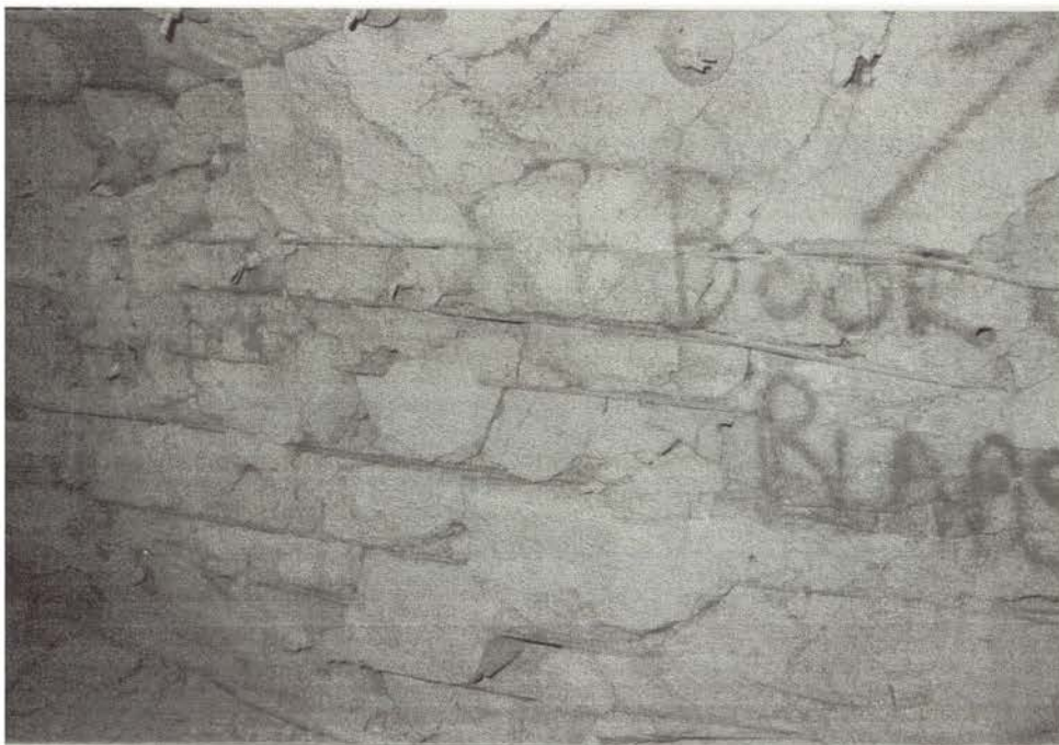
P.A. 3. DS2 on Damage Scale. Extensive cracking of rigid shotcrete lining in Tuffisitic Kimberlite Breccia on 630 metre level (RMR 50) after abutment stress has passed overhead.
