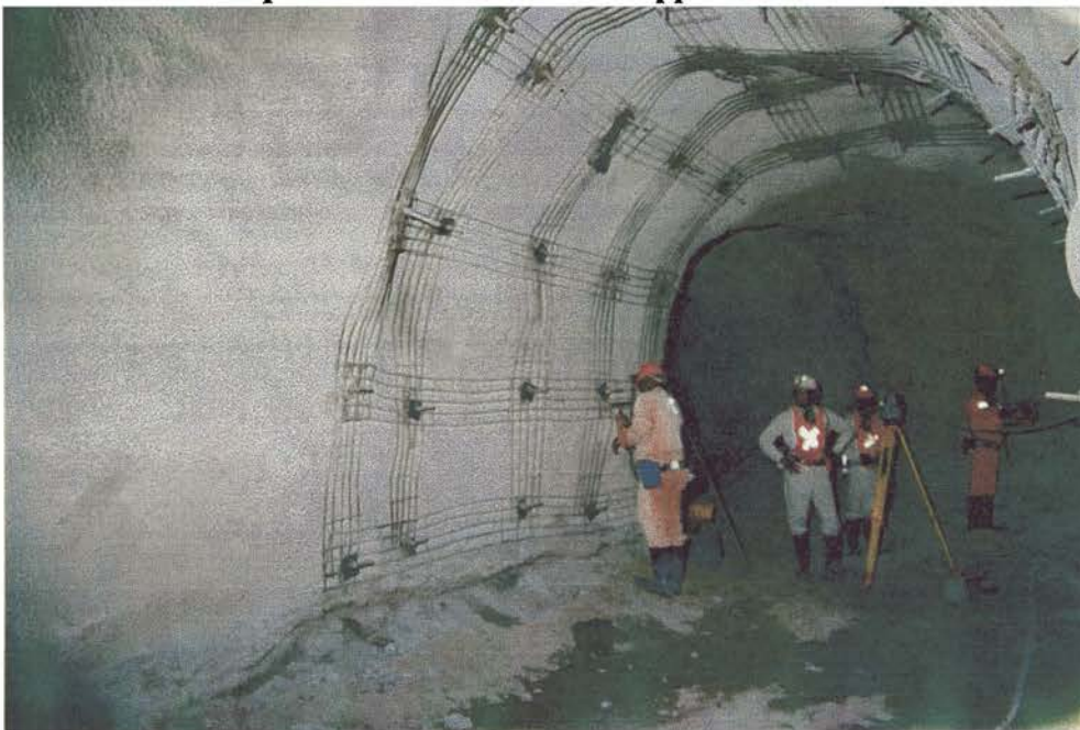
P.5.2. Drawpoints were supported with two layers of mesh and 2 layers of steel tendon straps tied into the sidewall by rockbolts. This steel construction was encased in 300 millimetres of shotcrete.
