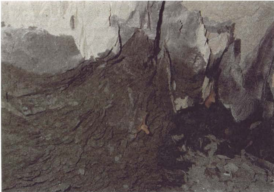
P.A..12. DS6 on Damage Scale. Decomposition of kimberlite results in ravelling and fallout of kimberlite around rockbolts with no damage to steel tendons or plate washers. Location;tunnel 117 on 601 metre level (RMR 53).
