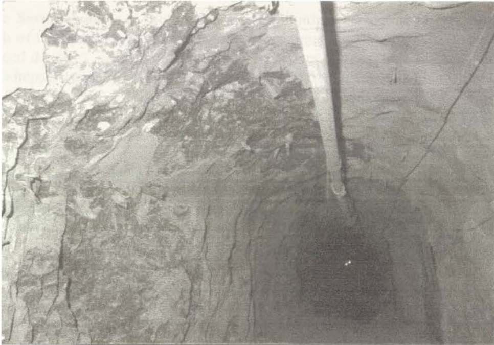
P.A.1. DS1 on Damage Scale. Shotcrete scaling in tunnel 21 on undercut level 30 metres from abutment (RMR 55).
