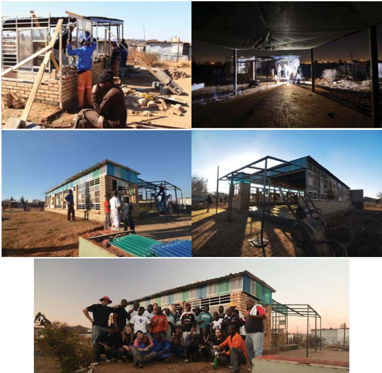
Figure 5.101: Conclusion of the construction process: team members including Honours architecture students, SPCDF members and JCP students under the auspices of 1to1 Agency of Engagement (Bennett 2012)
