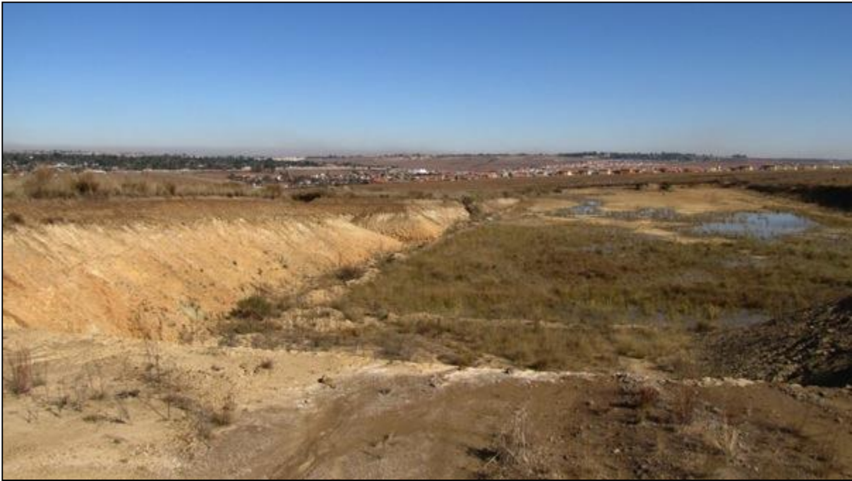
Figure 11. View towards the south showing the excavation and wet conditions during the dry winter months (June 2011).
