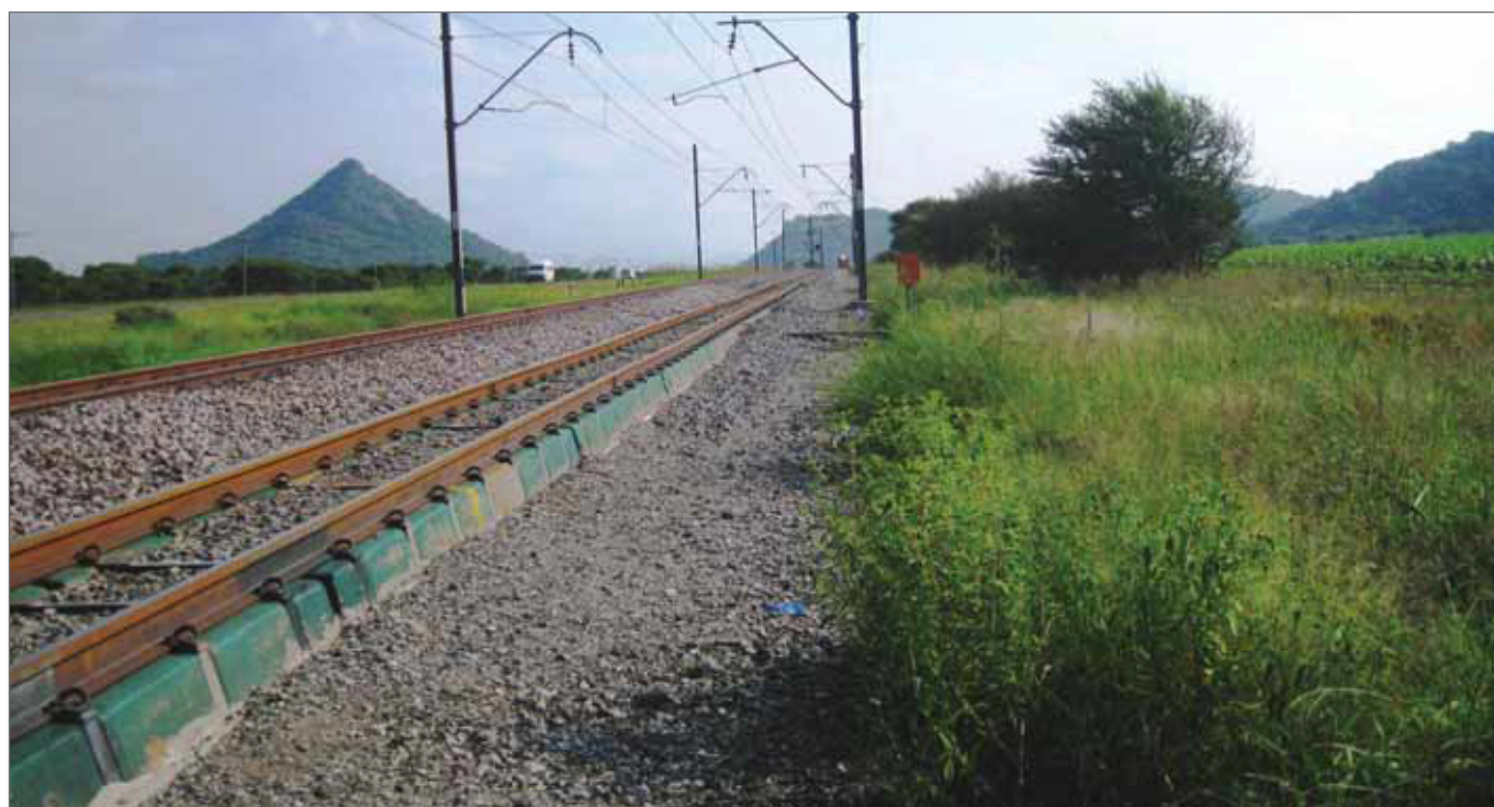
Figure 1: The test site was located at a Tubular Modular Track section of the railway line at the Amandelbult test site near Northam in Limpopo
