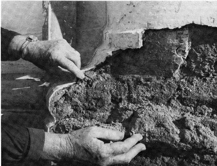
Old lime plaster and original 19th century moulding of corner pilasters were revealed when disfiguring cement overlay was removed.
