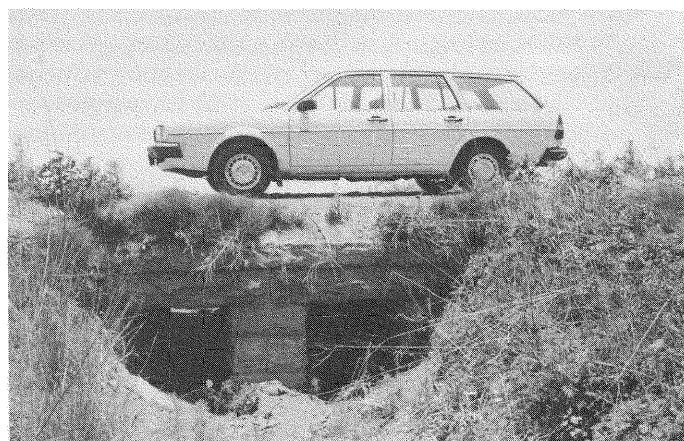
NZASM culvert of the rectangular type, i.e. with parallel walls supporting stone slabs and sheets of corrugated iron. In this particular case the culvert once formed part of an old embankment which was later turned into a road. (Photo: the author)
