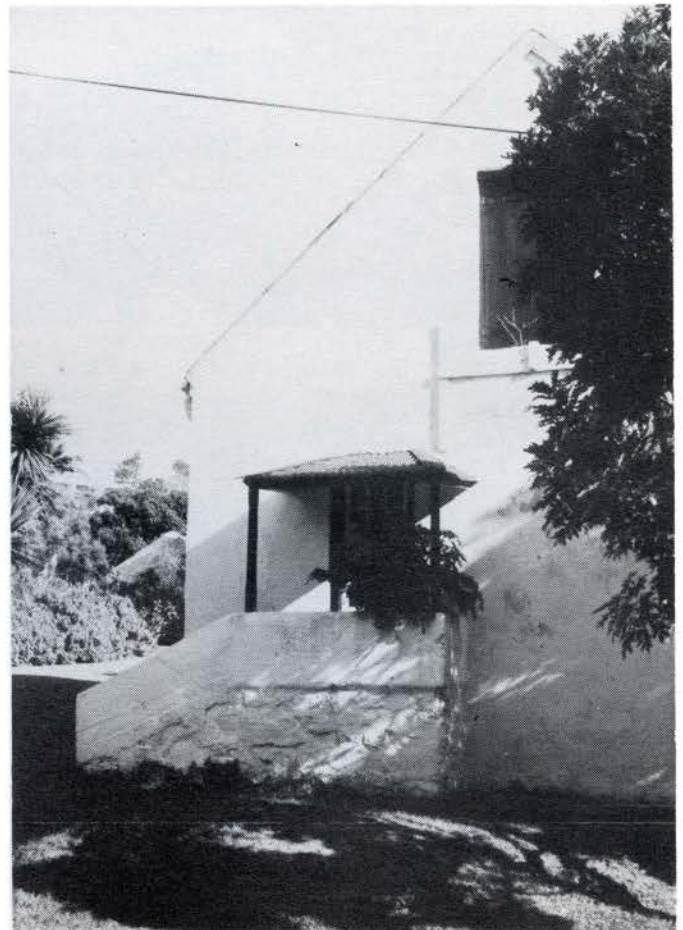
The door in the east wall of the house, thought to have been the original main entrance.
