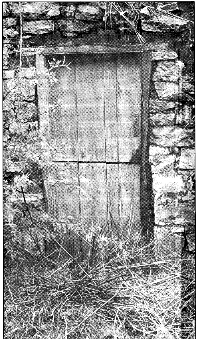
Detail: Back door with brass catch. The door frame of Vaal River Yellow Wood, the door panels of soft wood, perhaps of a later date.
