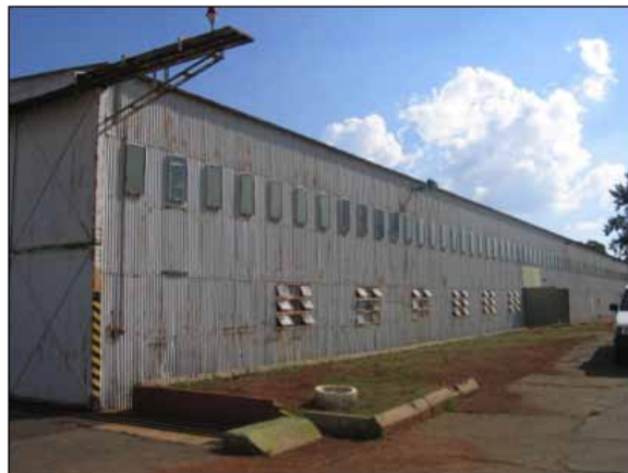
Figure 16 View of the side elevation of a Bellman hangar with the addition of small windows breaking the monotonous flat wall (photograph: M. Naudé).
