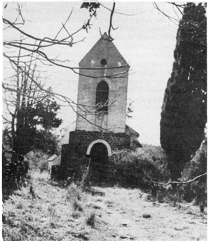
Frontal view of the Mission Church. This link with missionary work of the previous century ought to be saved.
