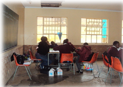
Photograph 2.2: Classroom with broken ceiling (taken 7-5-2012)
