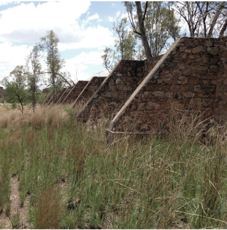
Figure:5_10. The heavy buttressed wall that runs along the western boundary of the compound. Notice the overhanging vegetation. (Author 2014)
