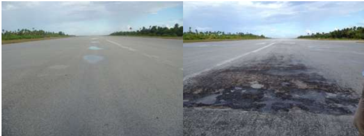
Figure 3: Surface condition of the Bonriki International Airport runway in South Tarawa. (L) Ponding, as a result of depressions. (R) Severe degradation of the surface, resulting from a basecourse layer failure and patching.
