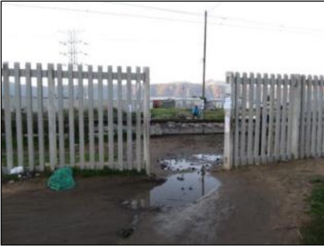
Figure 9(a): Opening in fence where NMT users illegally cross the rail reserve
