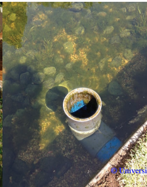
Figure 8.27 skimmer in fresh water pool
