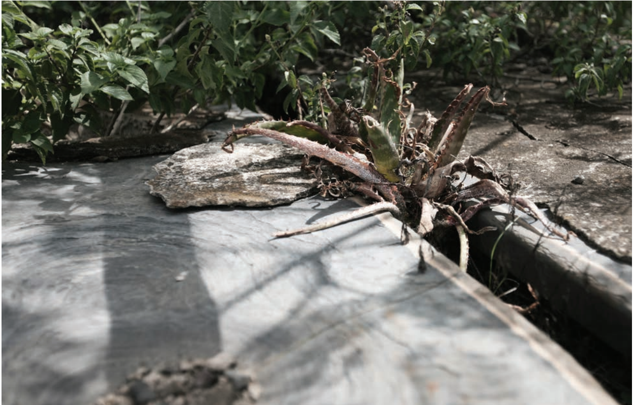
Figure 2.23 Aloes free to grow from an existing concrete wash abluition (2014)
