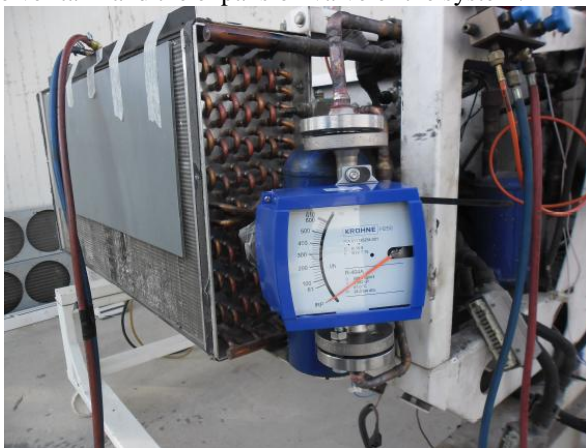
Figure 4 Flowmeter installation for refrigeration system
