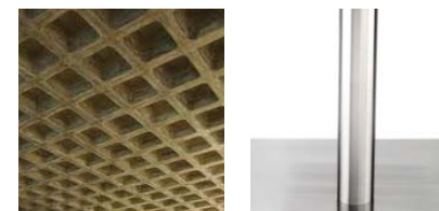
Fig. 10.11 Phase 1 structure: concrete coffer slab, round concrete columns clad with stainless steel plates for reflective effects
