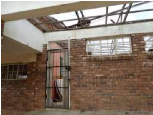
Photograph 3: Evidence of storm-damage to the roof of a remote partner-school (Mpumalanga Province, August, 2013).
