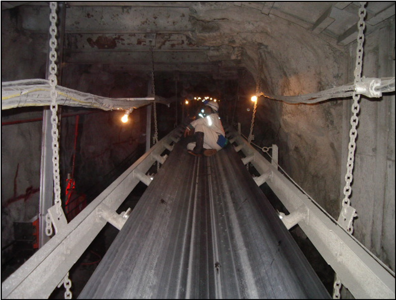
Figure 1.4.3a: Underground conveyor belt personnel transportation (BRPM, 2008)
