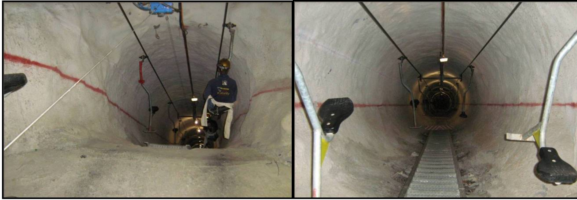
Figure 2.8: Chairlift installation in the raise bore shaft at Kopanong Mine (Kopanong Mine, 2008)
