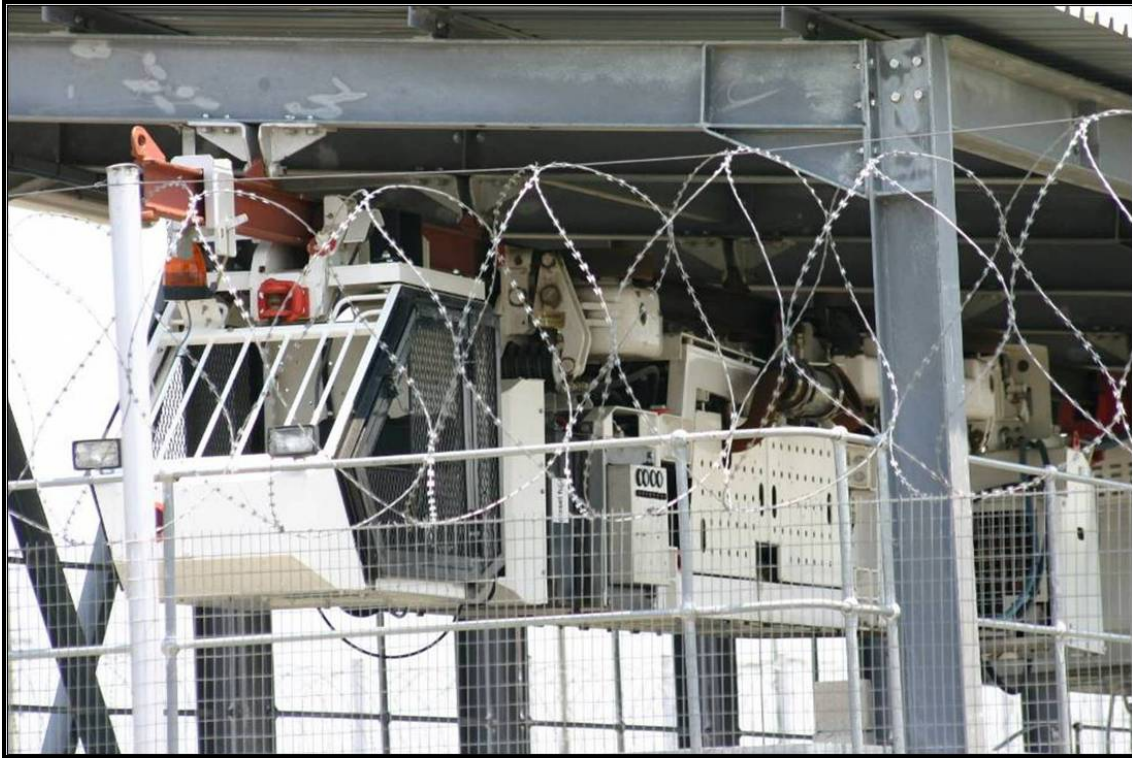
Figure 2.7a: Monorail Transportation System Infrastructure (AAP Union Section Mine, 2008)
