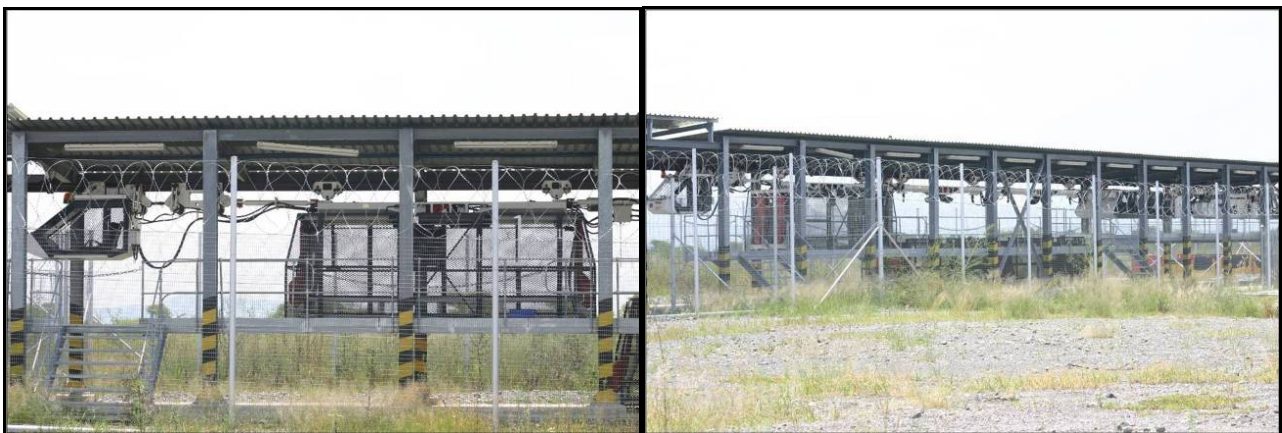
Figure 2.7: Monorail Transportation System Infrastructure (AAP Union Section Mine, 2008)
