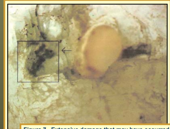
Figure 7. Extensive damage that may have occurred from the action of pitting
