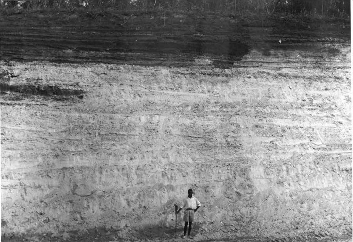
Plate 1. Soil profile exposed by bulldozing in preparation of the site of the Nokeng-e-Chweu Dam in Rosendal. Note the well-decomposed underground layer of saprolite below the darker soil layer.
