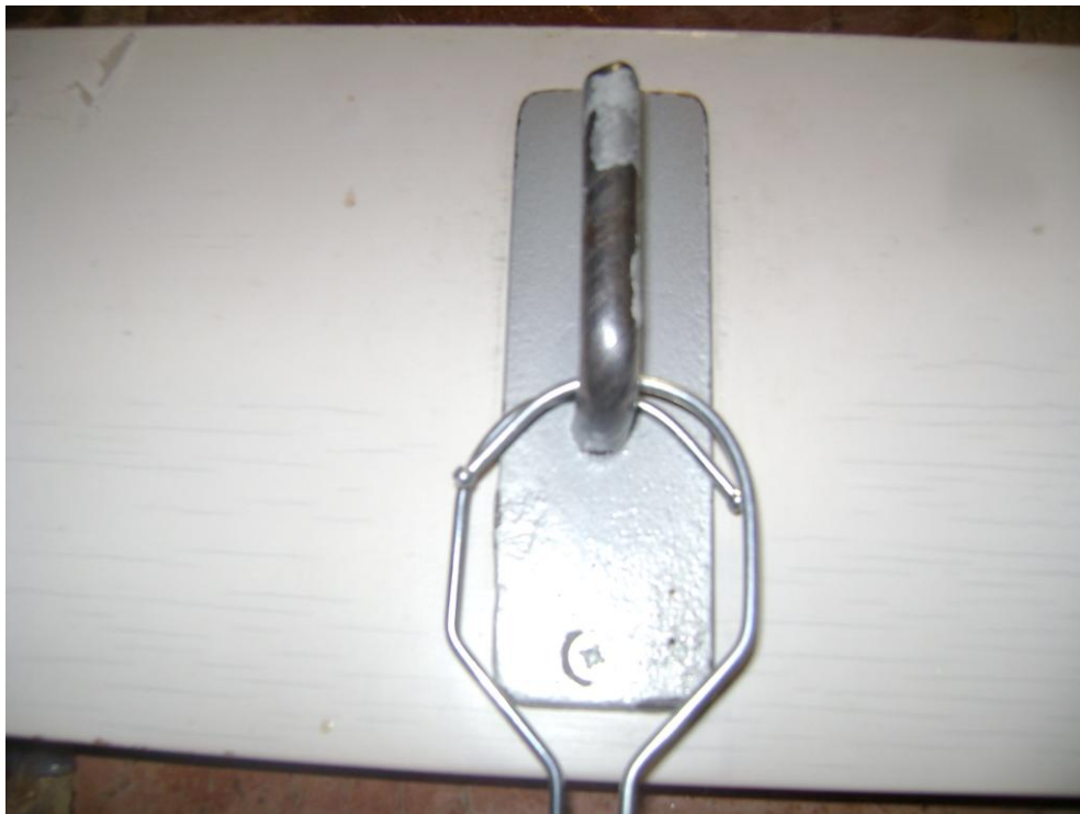
PHOTO 12: HANGING HOOKS NOT MAINTAINED IN HATFIELD PLAZA (P10:7)
