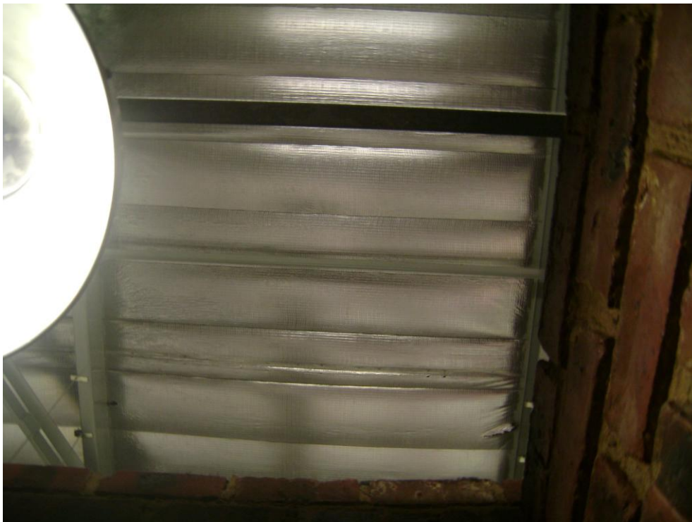
PHOTO 4: CUBICLE'S CEILING IN HATFIELD PLAZA (P6:7)
