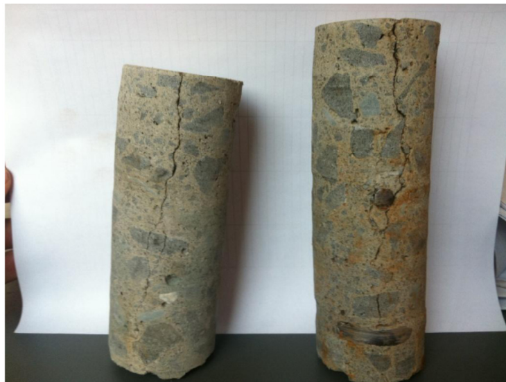
Figure 30: Cracks in the raft as indicated on cores taken form the raft (done by the main contractor)
