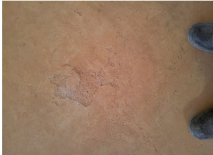
Figure 26: Delamination of the concrete surface (Photo taken at Kemach JCB by the main contractor)
