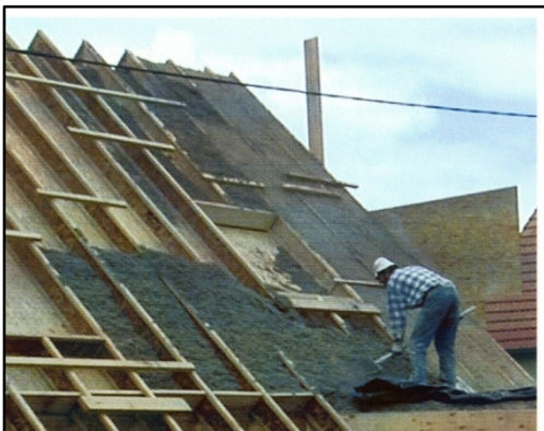
Figure 4 Hempcrete applied as a roof by making use of shutter boards. (Allin, 2012)
