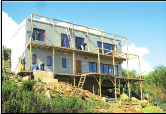
Figure 19: South Africa's first hemp home in Noordhoek, Cape Town during construction ( www.hemporium.com , 2012)
