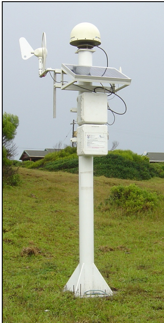
Figure 16. GNSS installation at Hamburg (HAMB), South Africa. This example station is totally self-contained. The station incorporates GPRS communication for data transfer, solar panel, wind charger, regulator and batteries for power, and a hermetically
