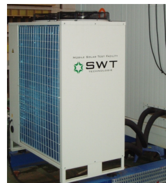
Fig. 3: Chiller connected to the container test facility
