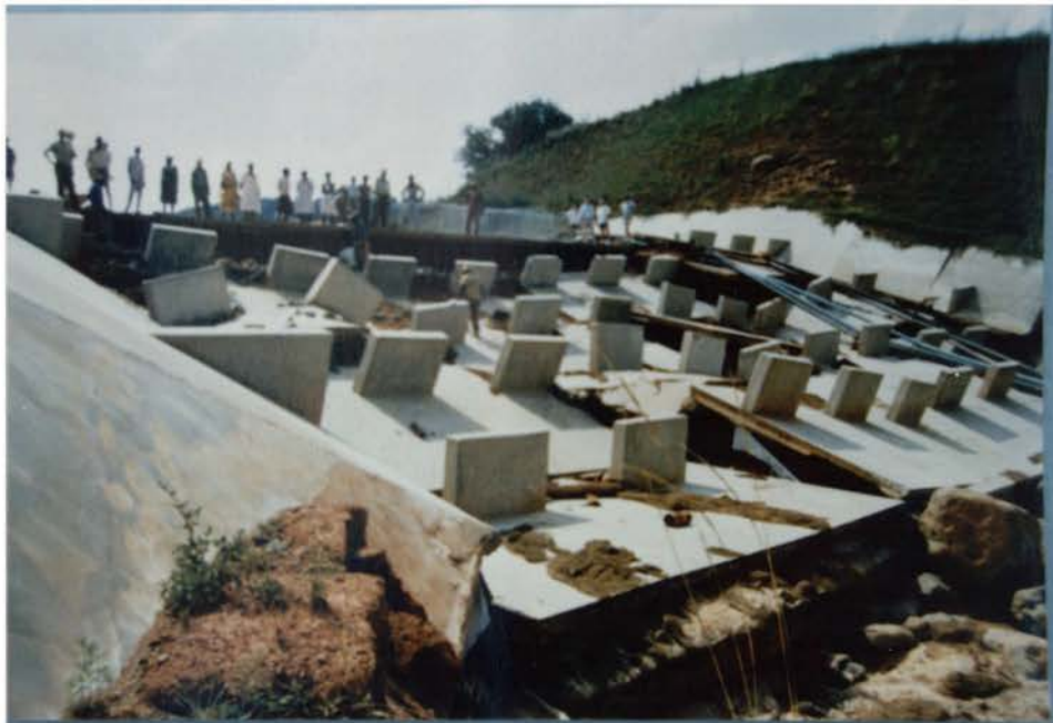
Plate 15 Damage to the spillway slab.
