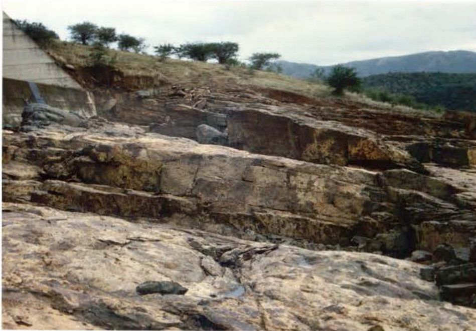
Plate 28 Extensive erosion of the jointed tillite downstream of the spillway (Van Schalkwyk).
