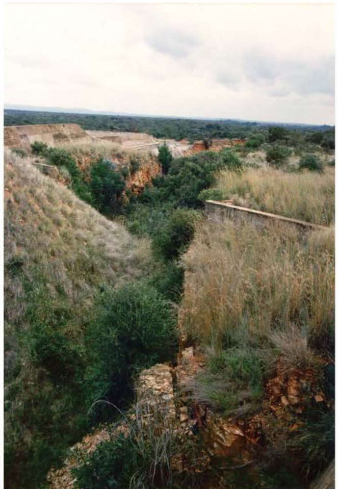
Plate 13 Old spillway structure which failed in 1936 after water discharge (Van Schalkwyk).
