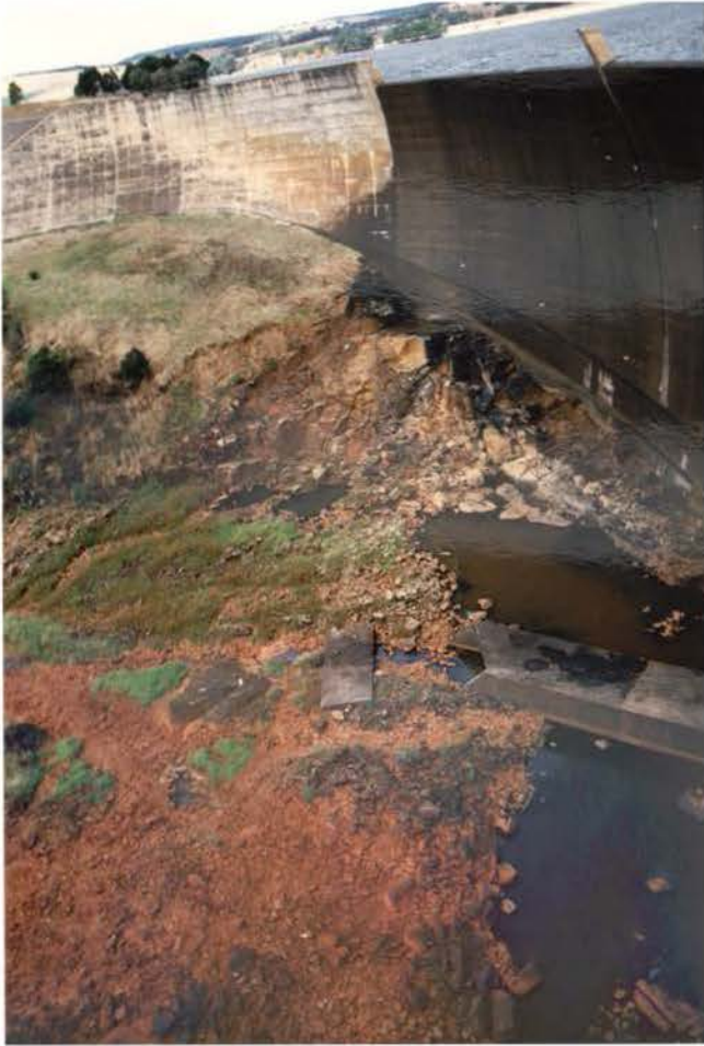
Plate 22 Removal of the topsoil downstream of the arch in the central and right flank areas (Van Schalkwyk).
