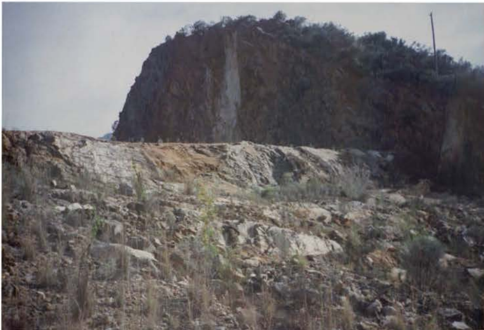
Plate 5 Extensively jointed rock mass with interbedded zones of clayey material on the flanks and in the floor of the channel.
