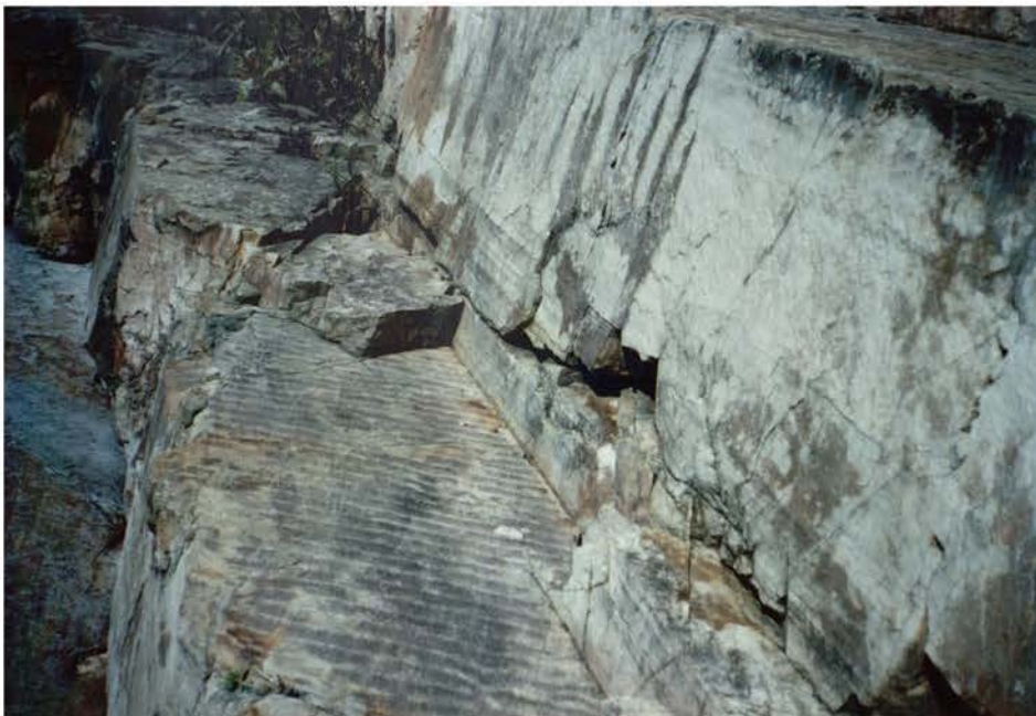
Plate 17 Steps and ridges in the spillway channel due to jointing
