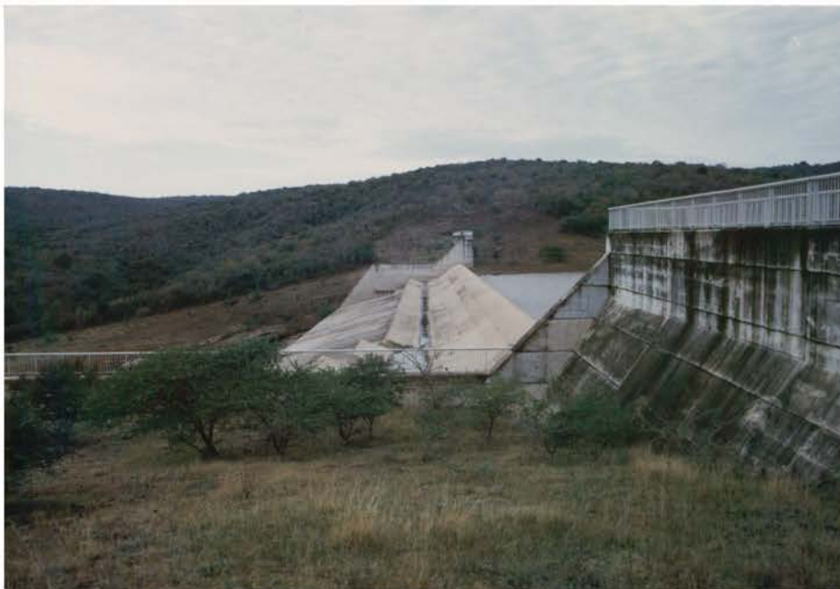
Plate 27 Goedertrou Dam - Side-channel spillway with flip bucket, apron and cut-off wall (Van Schalkwyk).
