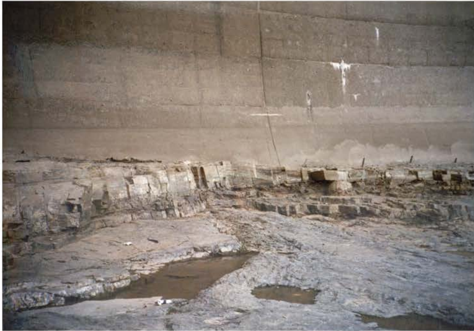
Plate 19 Jointed shale overlying dolerite rock mass downstream of the right spillway arch.
