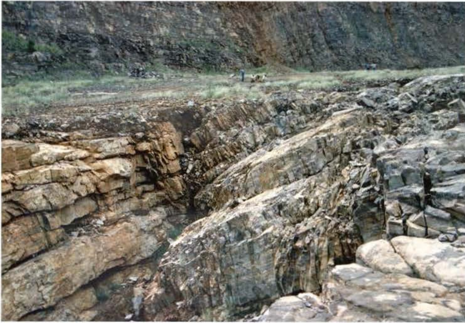
Plate 9 Scoured gorge in the spillway channel, closely related to the faults occurring on the right wall (Van Schalkwyk).
