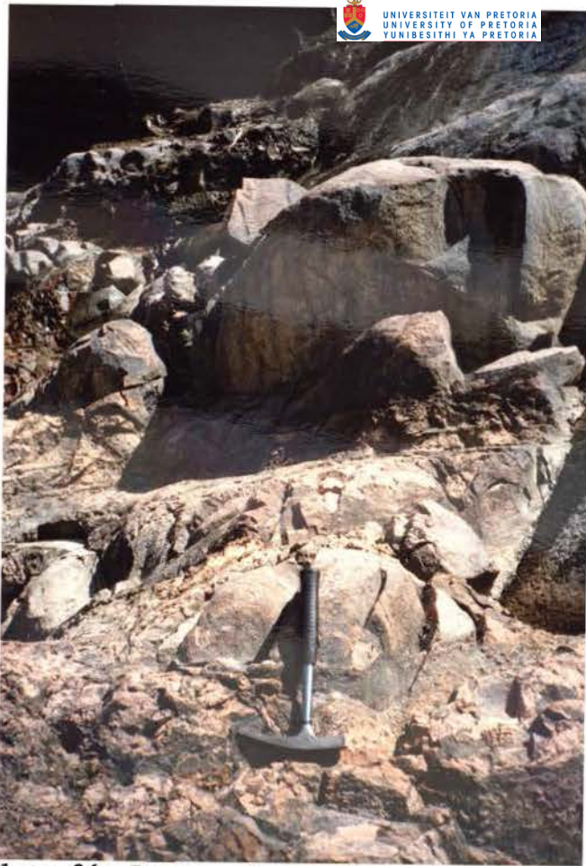
Plate 26 Zones of weathered felsite including unweathered jointed rock on the left side downstream of the arch.
