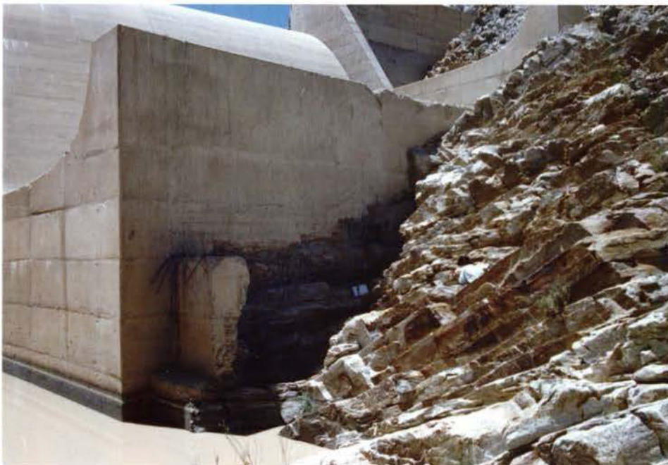
Plate 33 Erosion of the quartzites downstream of the bottom flip bucket (Van Schalkwyk).
