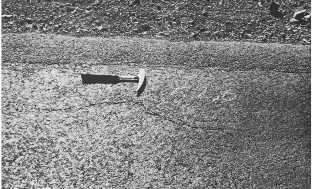
PHOTOGRAPH 16: Km 52,6 - Longitudinal cracking
