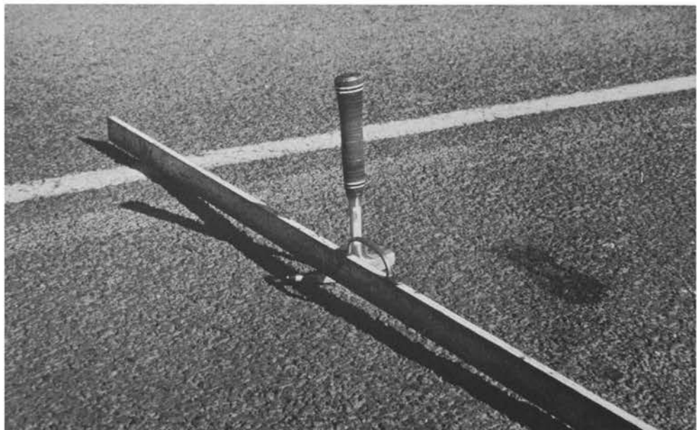
PHOTOGRAPH 15: Km 52,6 Rutting as a result of subgrade deformation is very evident in this section
