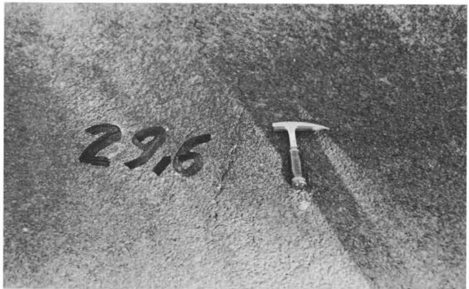
PHOTOGRAPH 4: Km 29,6 A typical transverse crack in the middle of a lane on Section 1C
