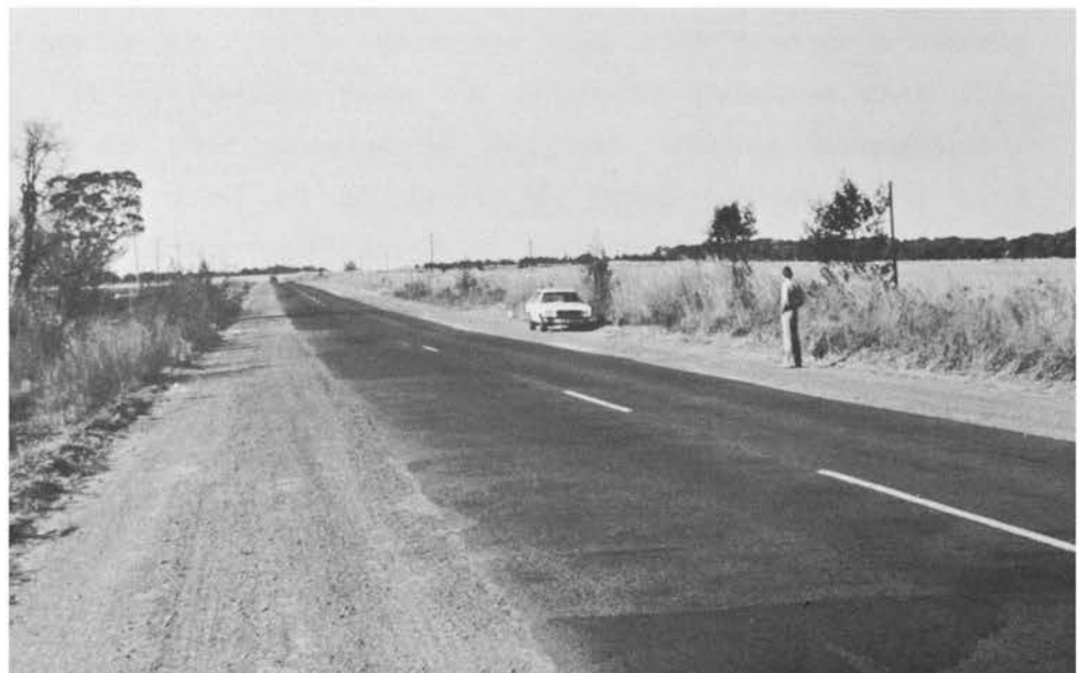
PHOTOGRAPH 12: Localized problem area Km 43,6 - km 44,3 - Patches and undulations clearly visible
