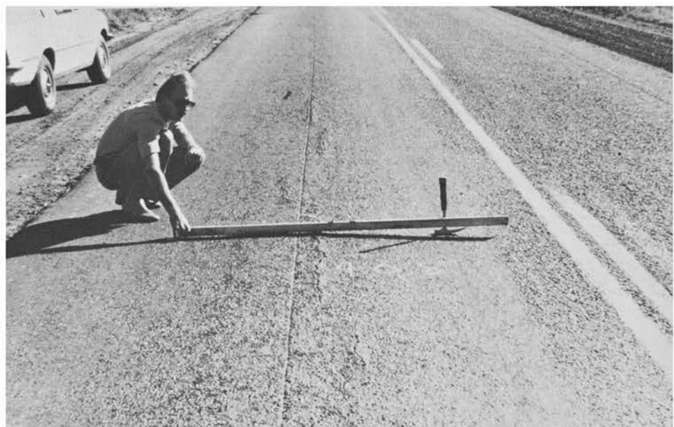
PHOTOGRAPH 14: Km 46,8 - Serious subgrade-associated deformation is evident in this section
