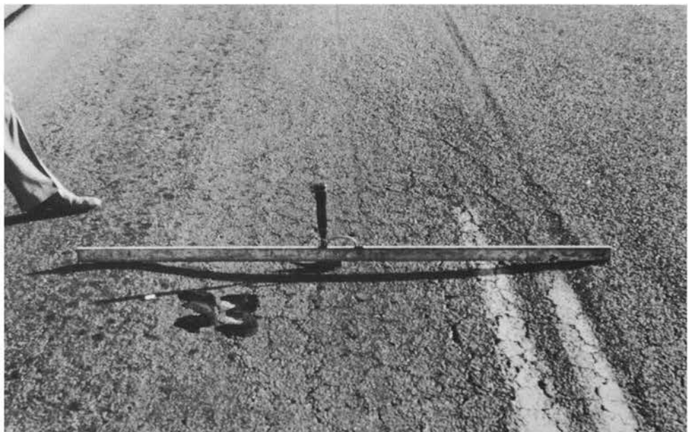
PHOTOGRAPH 6: Km 33,60 - Wide rutting with crocodile cracking indicating subgrade deformation
