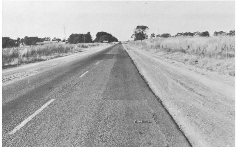
PHOTOGRAPH 8: Km 39,6 - Extensive patching with severe distress evident.
