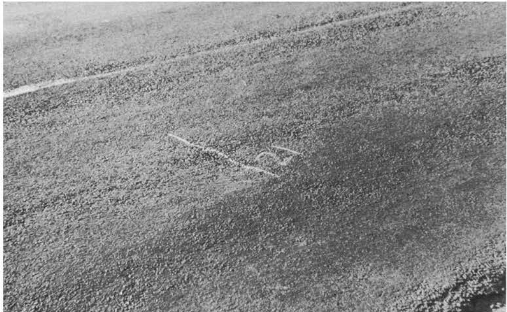
PHOTOGRAPH 2: Km 21 - Typical transverse crack shown with trafficking closing the crack in the wheelpaths (Section 1A)
