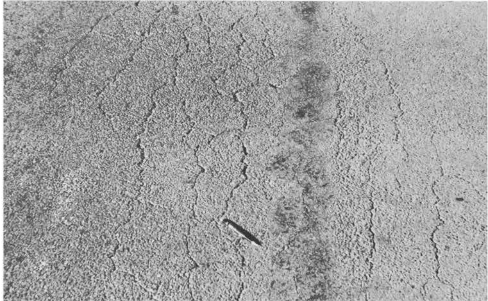
PHOTO .PH 13: Km 43,6 - Close-up of the surface of the road in Photograph 12, showing severe crocodile cracking
