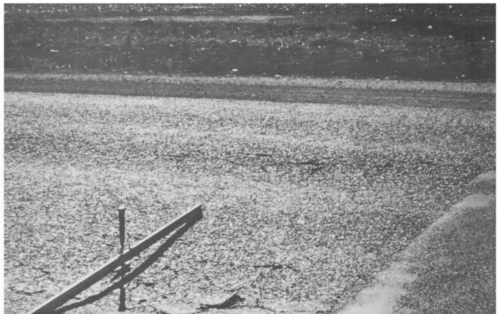
PHOTOGRAPH 11: Km 44,2 - Severity of the distress in this section is clearly shown by the rutting, patching and cracking patterns
