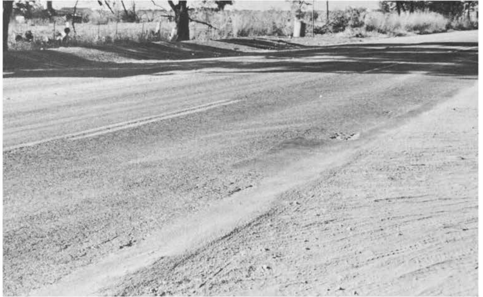
PHOTOGRAPH 10: Km 40,0 - Extensive patching, rutting, cracking and breaking up of the surface
