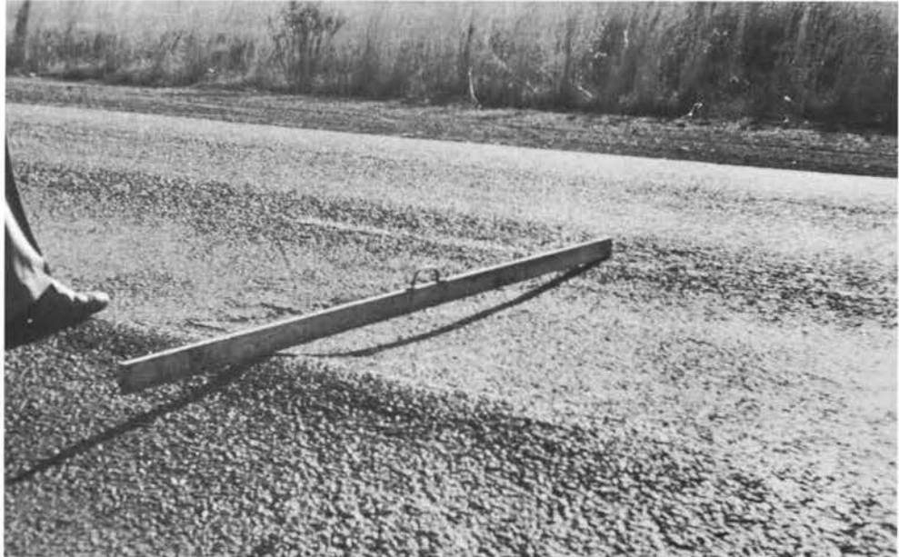
PHOTOGRAPH 3: Km 28,7 - Serious distress in the form of pavement layer failure is very evident in this section
